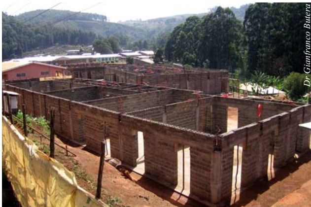
Figure 3. The Shisong Cardiac Centre is now under construction, and its inauguration is scheduled for November 2007.
